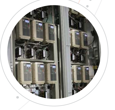
DDC Controls by Nortek Air Solutions Venmar used on the EnergyPack solution
