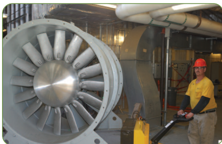
Existing 250 hp fan was a single vaneaxial type similar to the one shown here.
