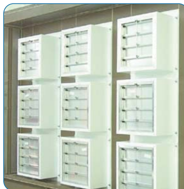
Discharge side of a 3x3 FANWALL array showing the backdraft dampers to isolate the fans when turned off.
