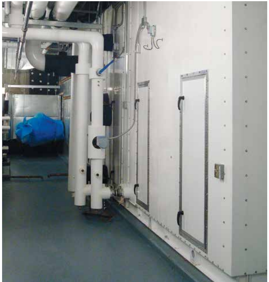
Even though they were brought into the mechanical room in piece parts, the installed Huntair® air handlers looked as if they had been factory-assembled.
