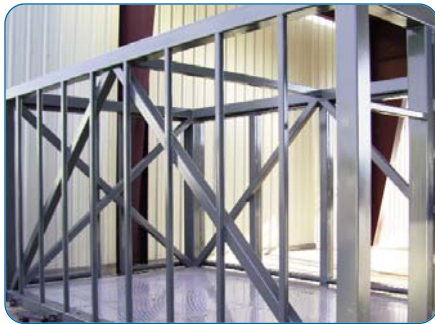
A custom steel skeleton was built by Governair for the air handlers, meeting the need to withstand winds up to 175 mph.
